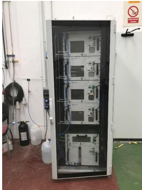
Figure 10: AEM electrolyzers installed at FHA facilities
